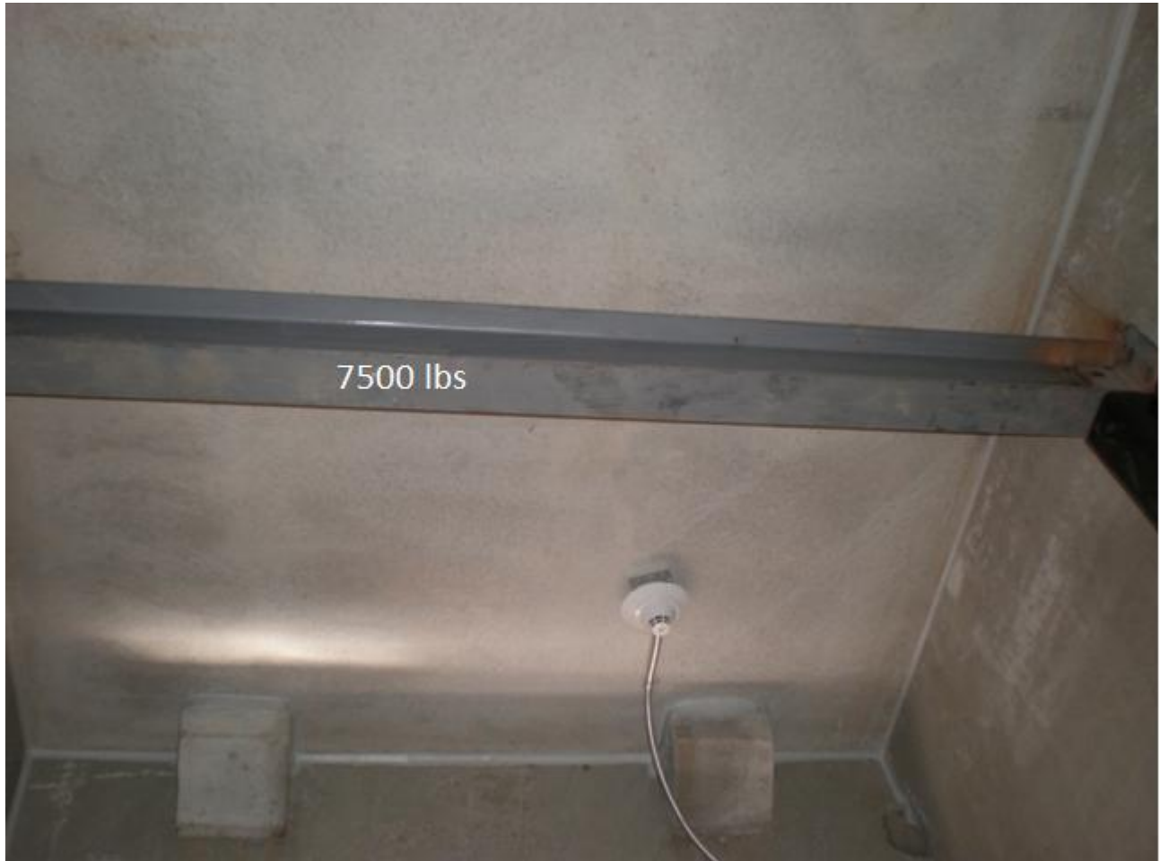
Example of "Hoist Beam"
